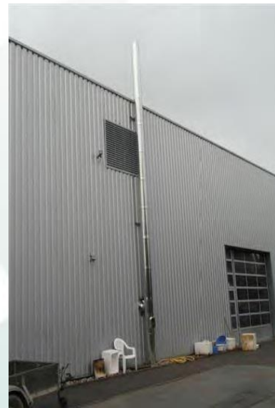
Extraction fresh air by 1 central duct and 1 inlet by a grating in the sidewall.
